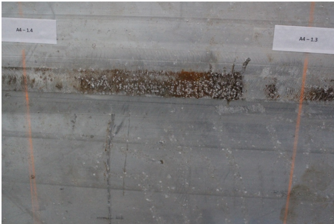
Figure 4: Corrosive Staining at Weld A4
