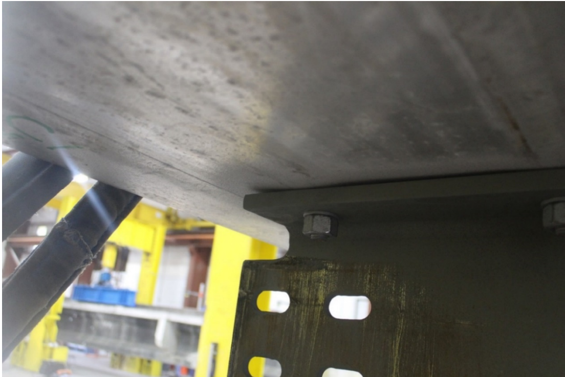
Figure 11: Gap between Steel Stringer and Generation I Aluminum Panel
