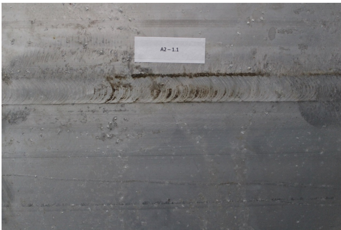
Figure 5: Corrosive Staining at Weld A2
