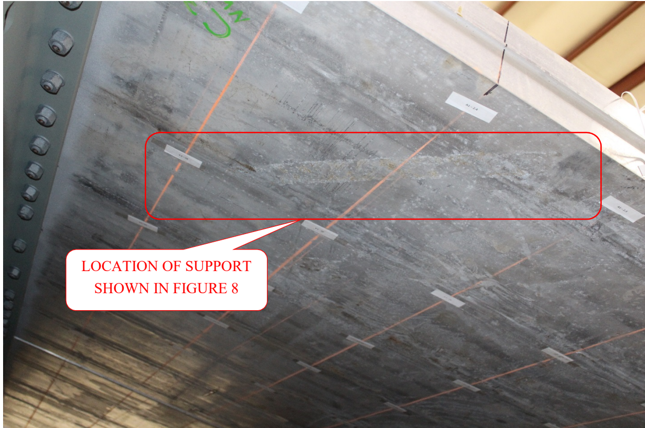
Figure 7: Corrosive Staining at Generation I Panel
