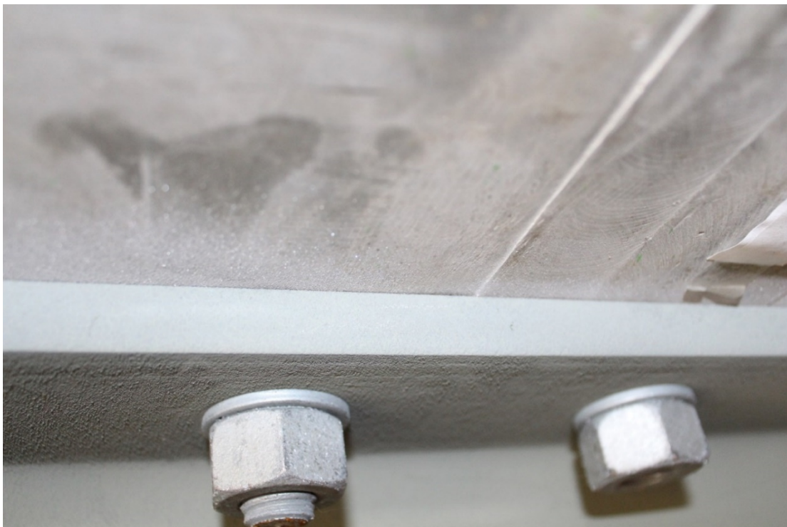
Figure 12: Gap between Steel Stringer and Generation II Aluminum Panel
