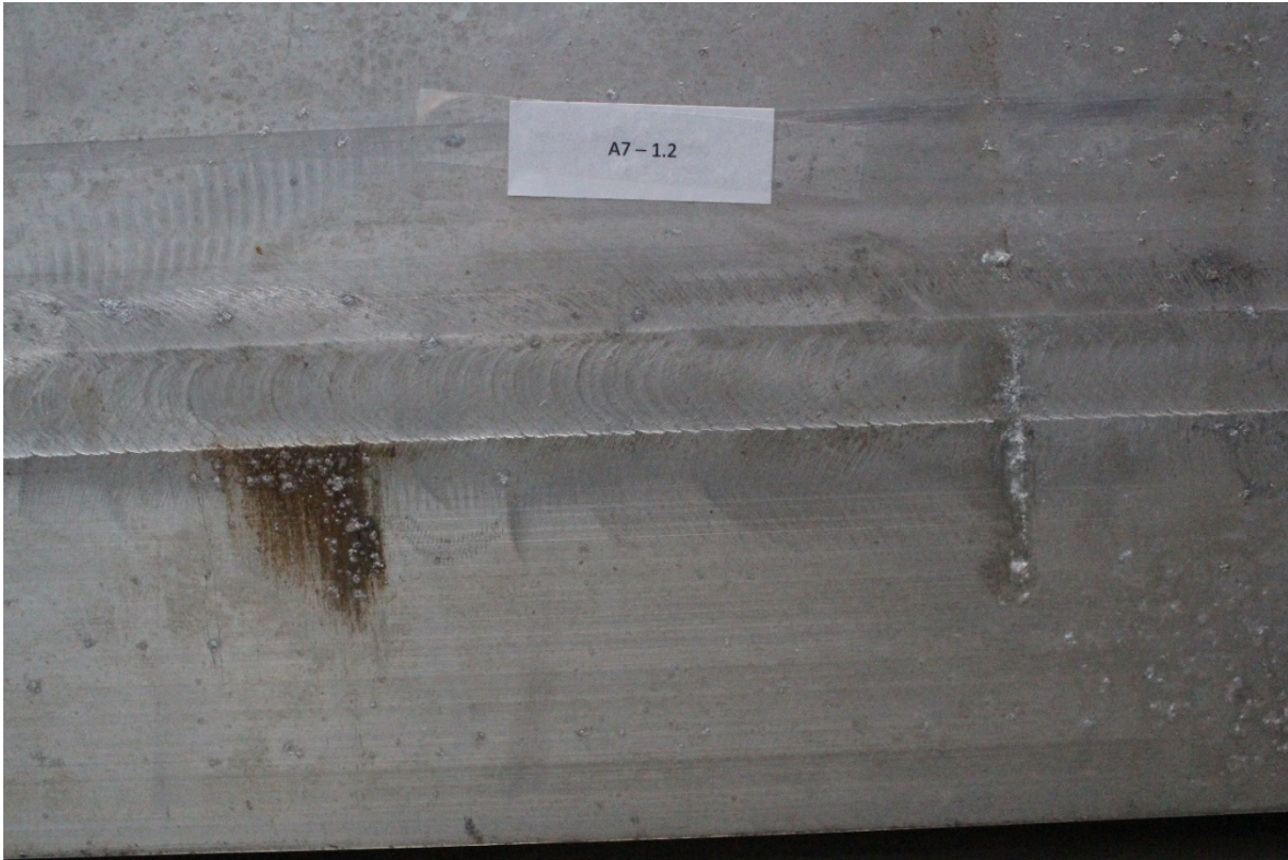
Figure 6: Corrosive Staining at Weld A7
