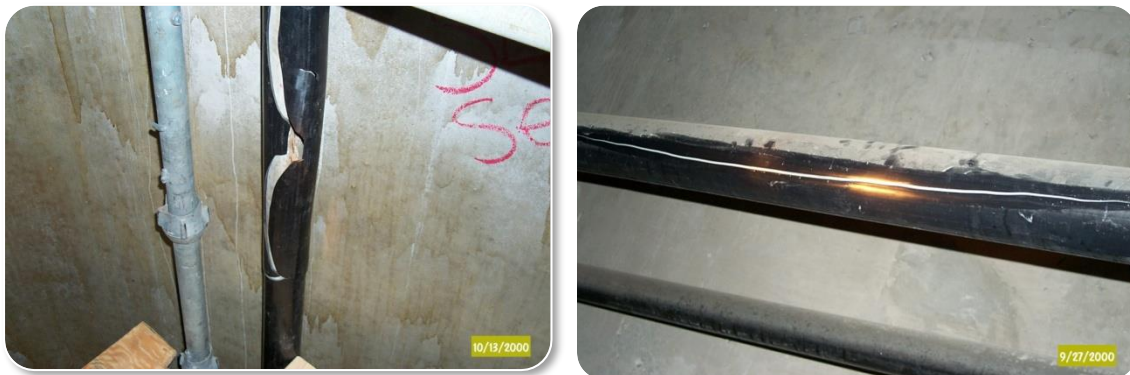
Figure 2-7: Examples of types of observed cracking of ducts.
