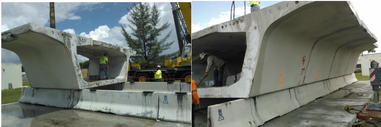
Figure 3-15: Photos taken during placement of first segment (left) and last segment (right).
