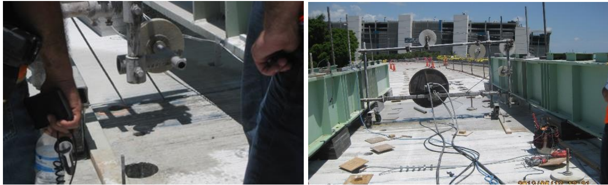
Figure 3-5: Wire saw cutting at middle of span 2 (left) and shear transfer beams (right).
