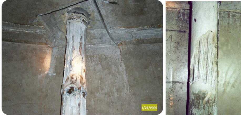
Figure 2-6: Corrosion activity in voided area (left) lack of corrosion activity in void area (right).
