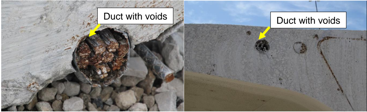
Figure 3-9: Some ducts were fully grouted, and some other ducts were partially grouted.
