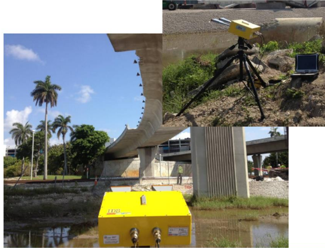
Figure 4-26: IBIS-S antenna shows system orientation and corner reflectors.
