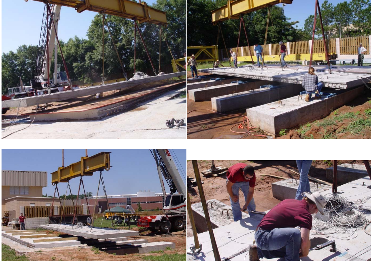
Figures 14 - Starting on the upper left and going clockwise: (a) Lifting the panels from the form; (b) Lifting; (c) Leveling; (d) Return Lift.
