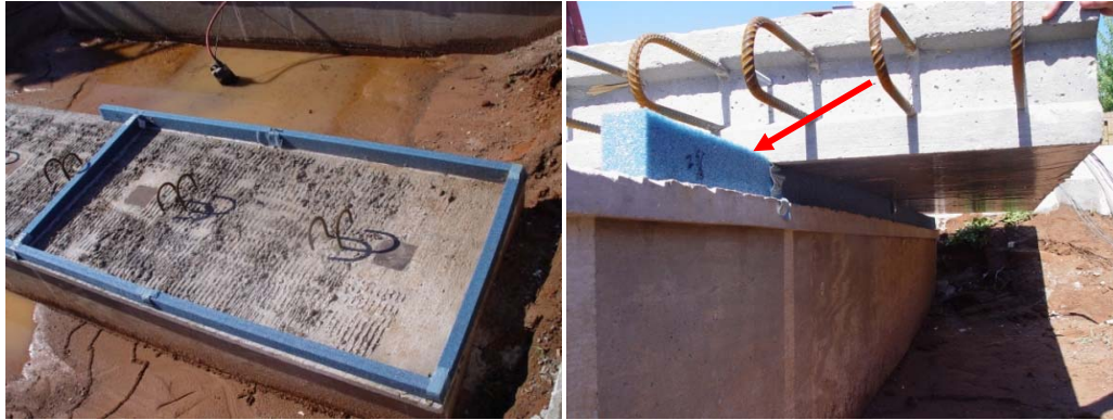
Figure 6 - Plan view of concrete beams with haunch forming material and shear reinforcement (Left); Side view of haunch forming material once panel is set (right).
