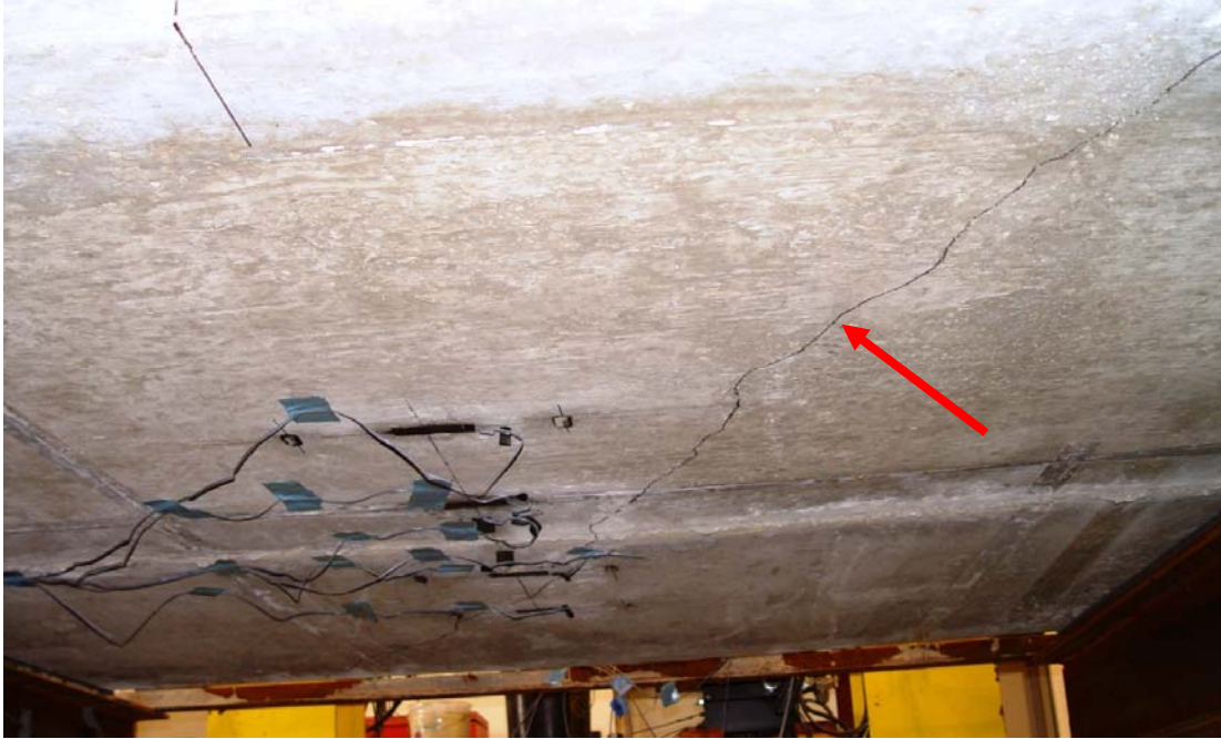
Figure 11 – Diagonal Crack after Continuous Load Test
