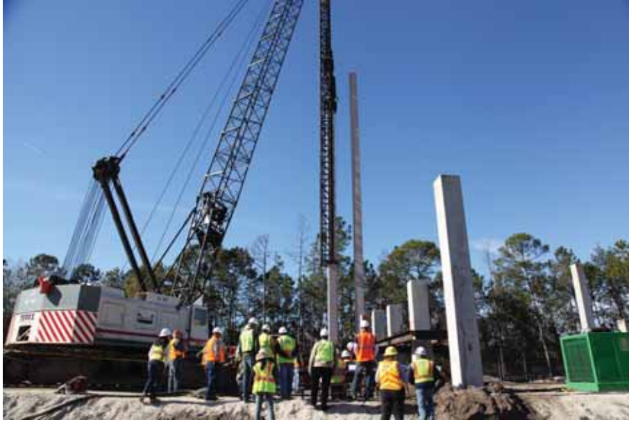
Figure H.31: End bent 3-1 on westbound bridge; Two 100-ft piles ready to be driven
