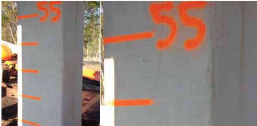
Figure 15 – Vertical Crack and Close up
