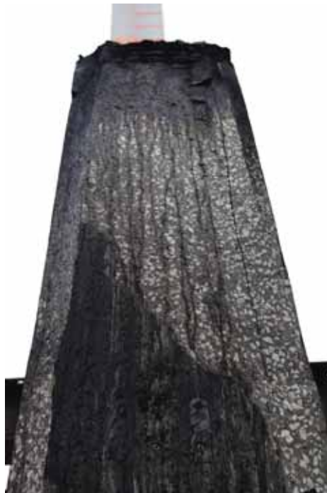
Figure H.34: Concrete spalling on head of Pile 1 after being driven
