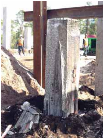
Figure 14 – Spalling near the Top of Pile N2
