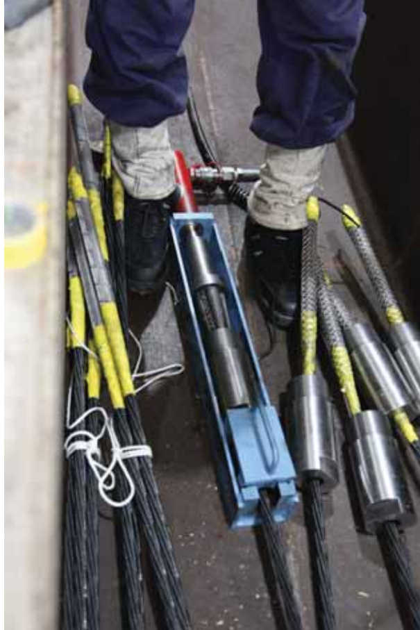
Figure H.13: CFCC coupler installation: pushing wedges into coupler with jacking system
