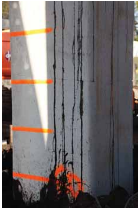
Figure H.38: Horizontal (tension) crack in Pile 2
