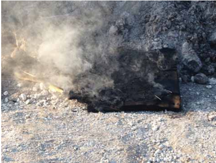
Figure H.33: Charred pile cushion, after Pile 1 driving
