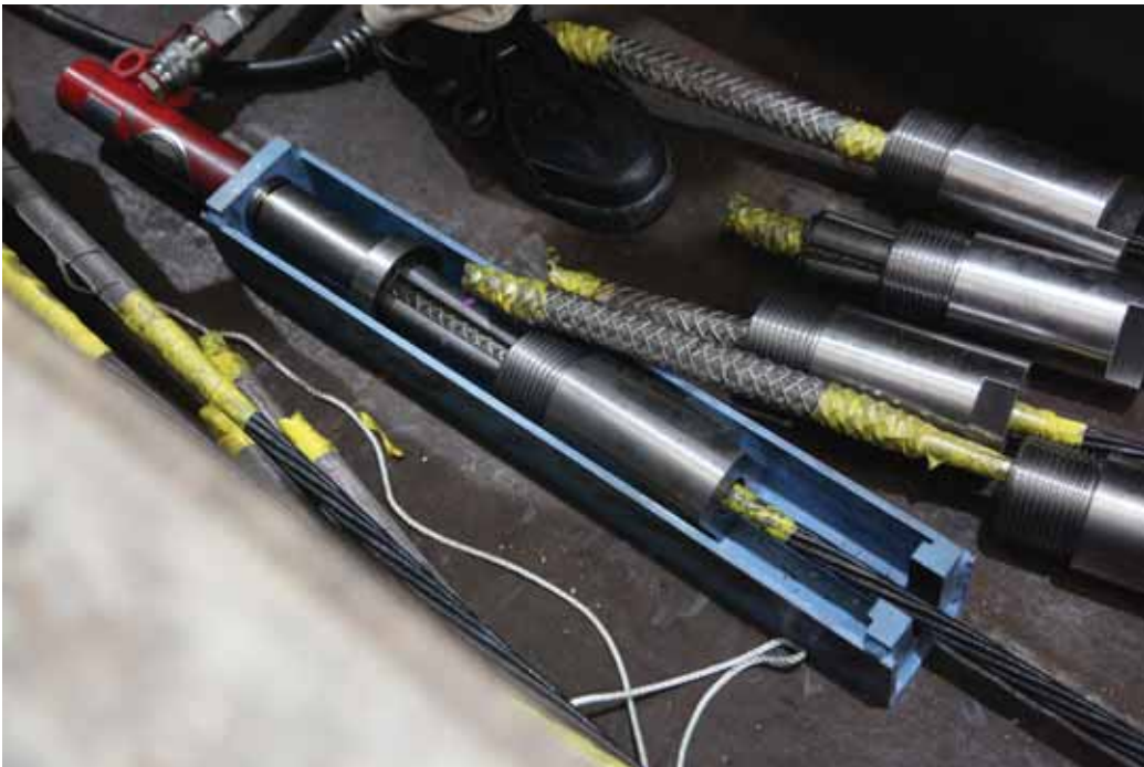
Figure H.12: CFCC coupler installation: coupler in jacking system, ready for pushing
