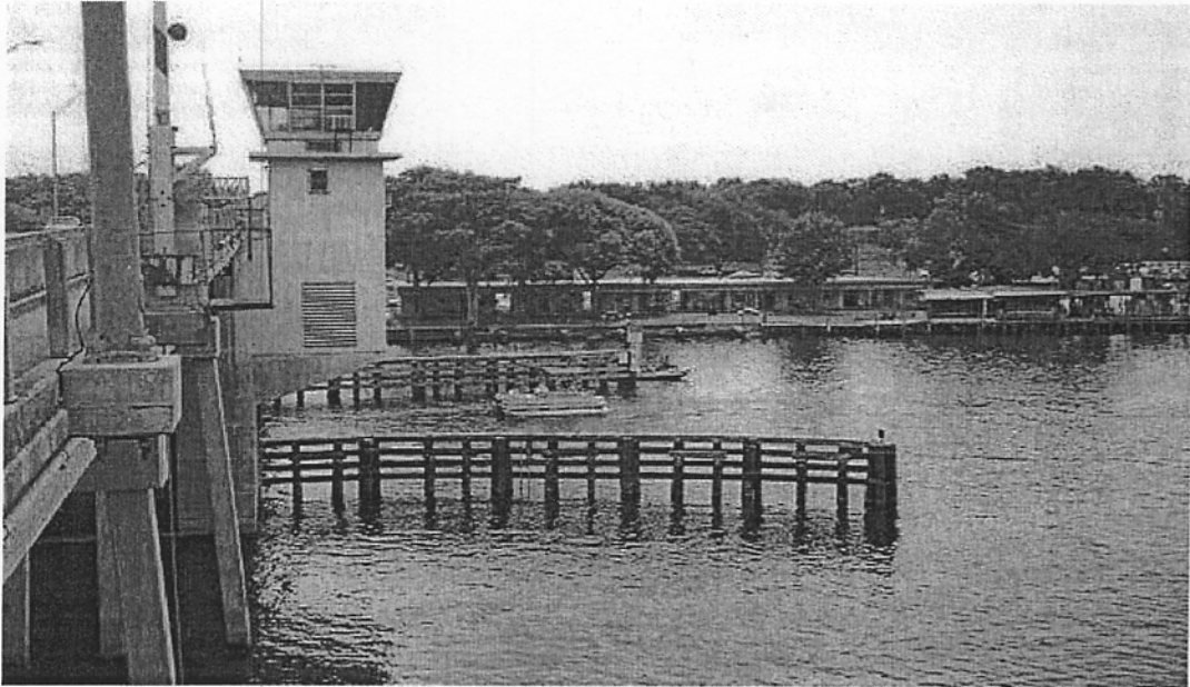
Figure 1.1. Fender Systems Currently Used by FDOT
