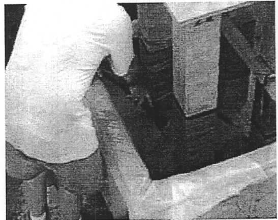
Figure 2.21 Filling Control Bed.
