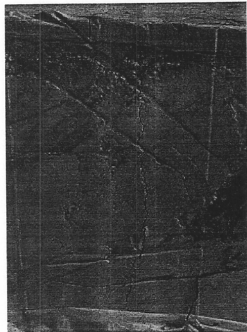
Figure 5.24 Vertical crack at edge of CIP seal slab.
