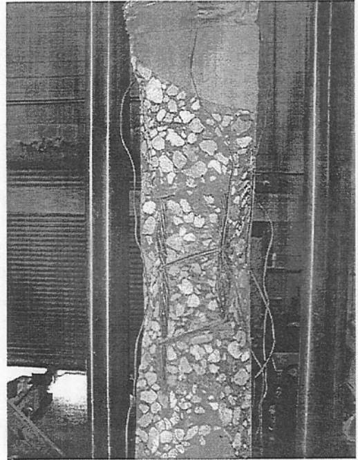
Close-Up of Damage
