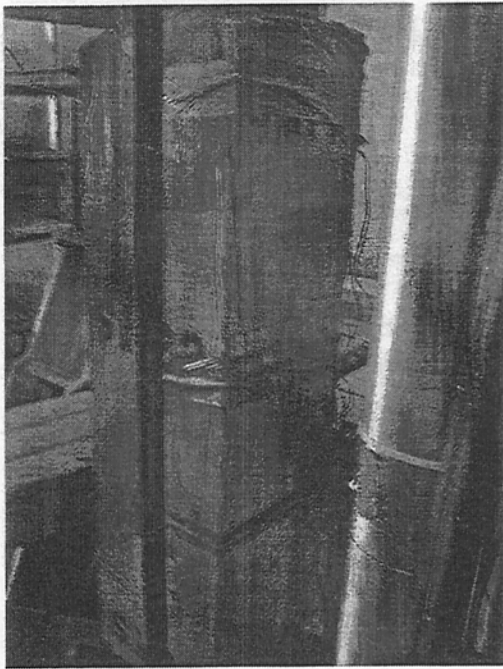
Note Splitting at Edges
