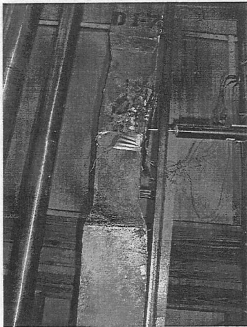
Close-Up of Failed Control
