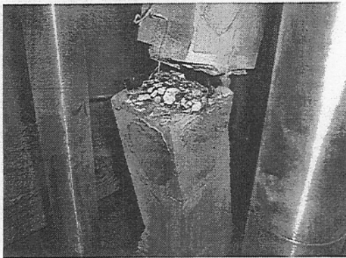
Control Fails in Two Pieces
