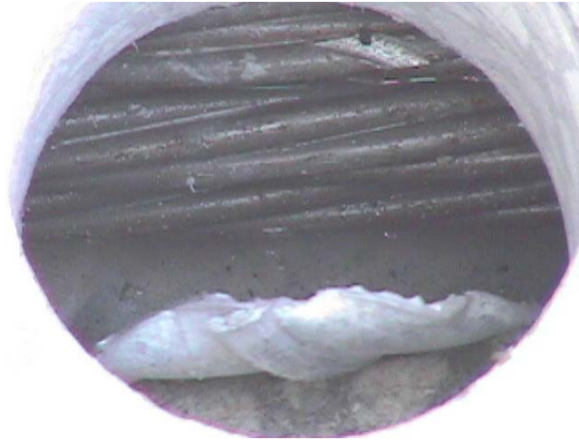
Figure 4.9 - Tendon 10, core drilled at Segment 54.
