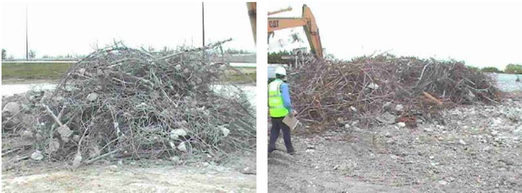
Figure 7.21 and 7.22 – Steel remains of crushed segments
