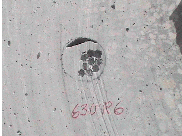
Figure 4.8 - View of duct with void
