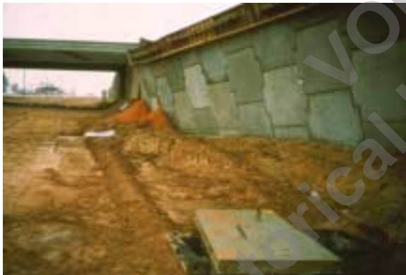
Figure 28, Wall Failure from Exterior Excavation
