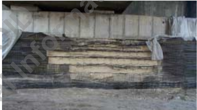
Figure 31, Fire Damaged Reinforcement
