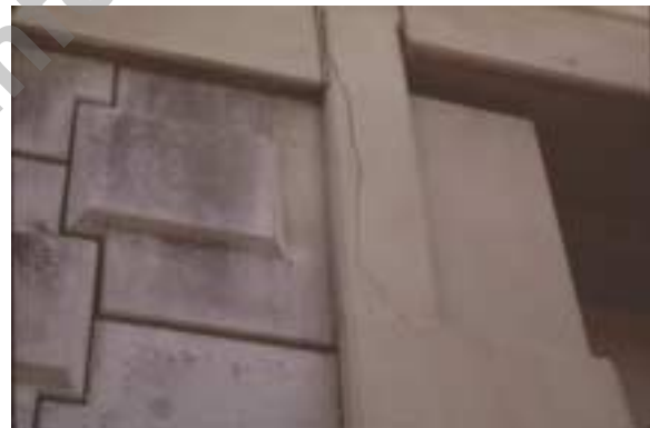
Figure 20, Tension Break in Cheek Wall
