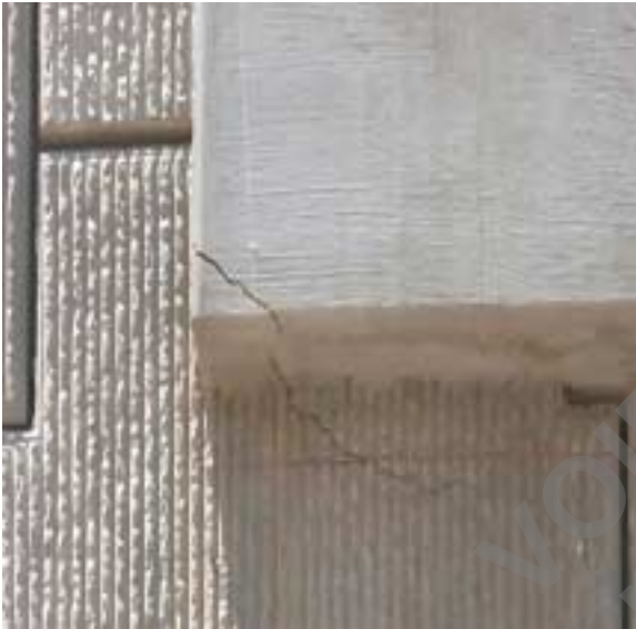
Figure 19, Cracked Panel and Cheek Wall
