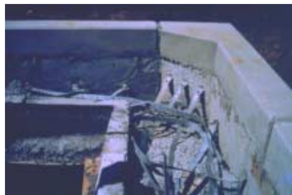
Figure 25, Not Proper Avoidance of Drainage Structure
