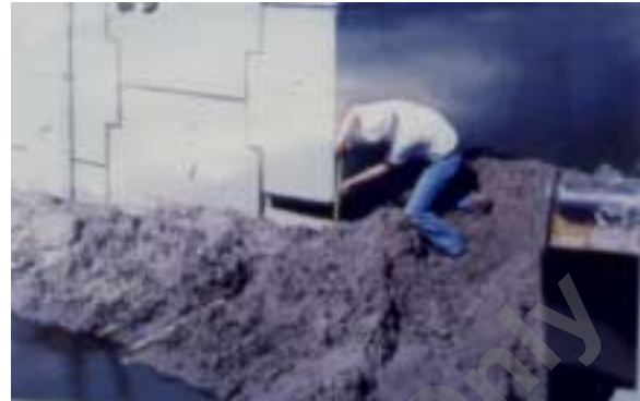
Figure 26, Settlement from Excavation
