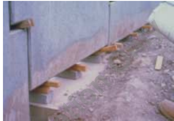
Figure 2, Improper Leveling Pad
