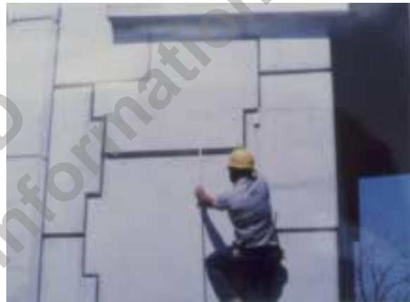
Figure 27, Joints Opening from Settlement
