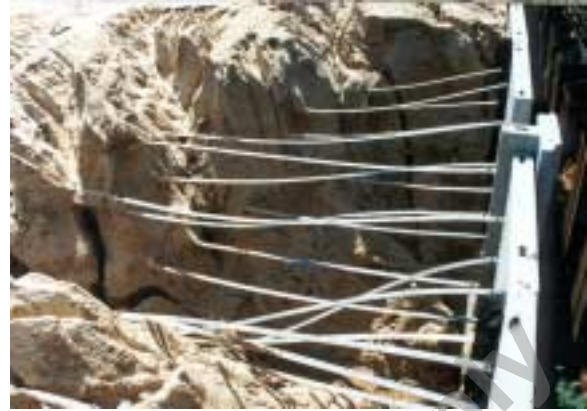
Figure 23, Wash Out From Around Reinforcement
