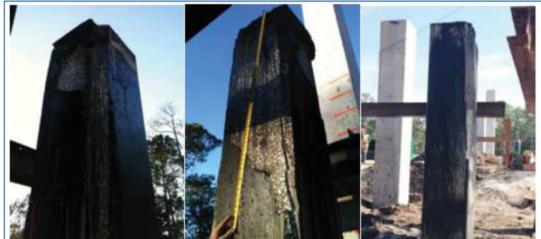
Figure 12 – Diesel Covered Pile with Spalled Sections
