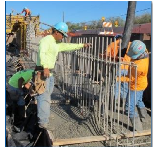
Photograph: GFRP Bars in retaining walls railing combination (Hughes Bros.)
