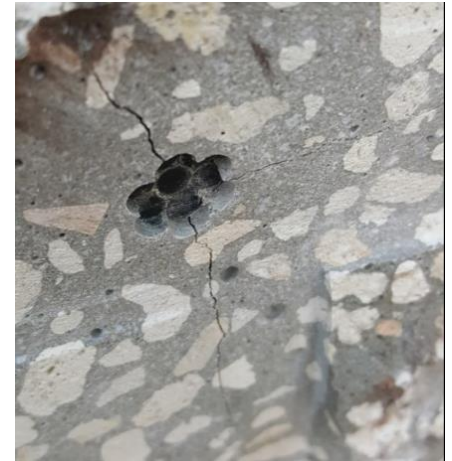
(Photographs - FDOT). Strand contraction and cracking at cut-off.
