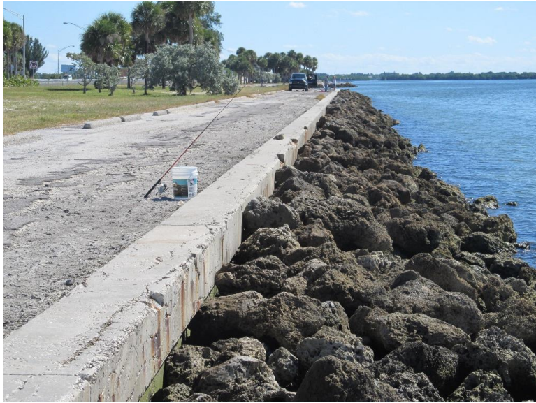
West Area – Damaged Seawall Cap
