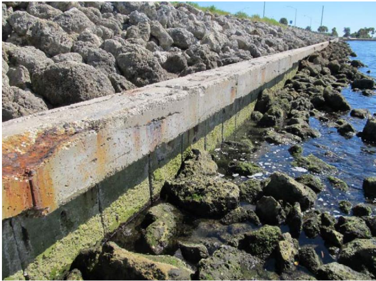
Northwest Area – Damaged Seawall Cap
