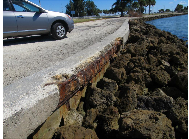
West Area – Damaged Seawall Cap
