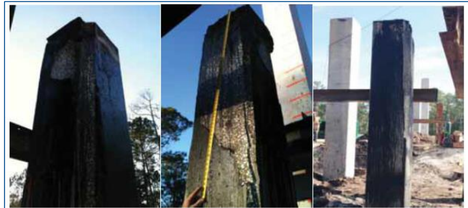
Figure 12 – Diesel Covered Pile with Spalled Sections
