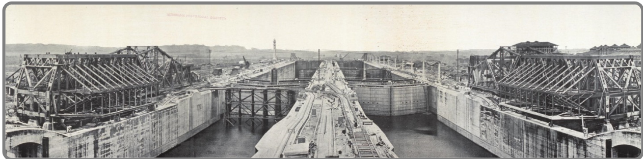
Source: Birds eye view of Gatun Locks construction, Panama Canal (U.S. Library of Congress, 1913)
