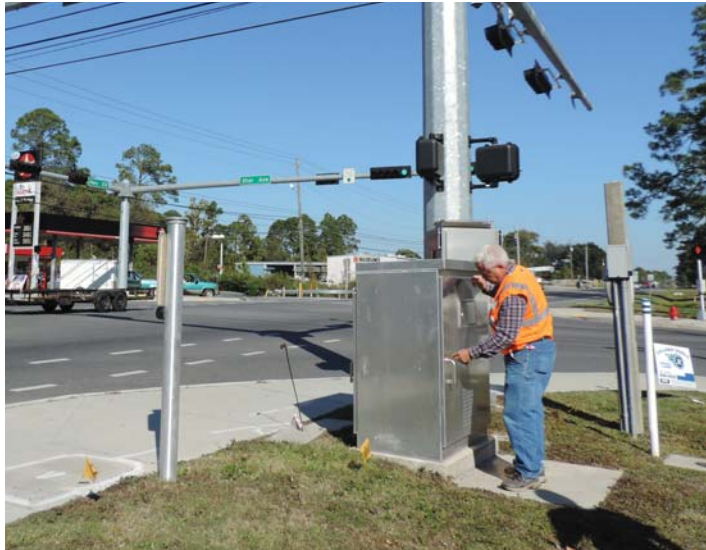
A worker accesses a traffic control box at a typical Florida intersection. These ubiquitous cabinets house Actuated Signal Controllers that control the traffic signals, pedestrian signals, and other electronic devices and are used to regulate both vehicular and pedestrian traffic at intersections.
