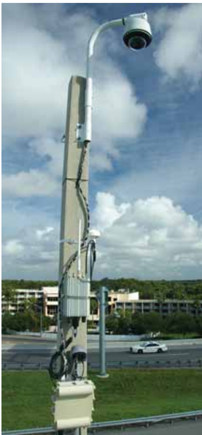
Advanced traffic management systems use a variety of intelligent transportation system technologies to manage traffic. A variety of equipment is mounted on this pole along the connected vehicle test bed in Orlando. From top: closed-circuit television camera; GPS antenna (small white object on the right side of the pole); road-side equipment, which transmits information from the vehicle to the regional transportation management center; microwave vehicle detector.
