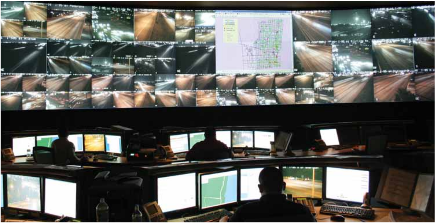
Florida's Regional Transportation Management Centers (RTMCs), located in major metropolitan areas, are the nerve centers for disseminating information about traffic conditions gathered with ITS devices to the traveling public and emergency workers. Pictured above, the Broward County/District 4 RTMC located in Fort Lauderdale, Florida, is staffed 24-hours per day, seven days per week, 365 days per year. Pictured above: RTMC operators in Broward County monitor closed-circuit television (CCTV) cameras deployed along I-95, I-595, and I-75 and post messages to dynamic message signs. When operators detect an incident, such as stopped or slowed traffic, operators dispatch road rangers and the severe incident response vehicle, in coordination with the Florida Highway Patrol (FHP), to determine specific incident and congestion locations.
