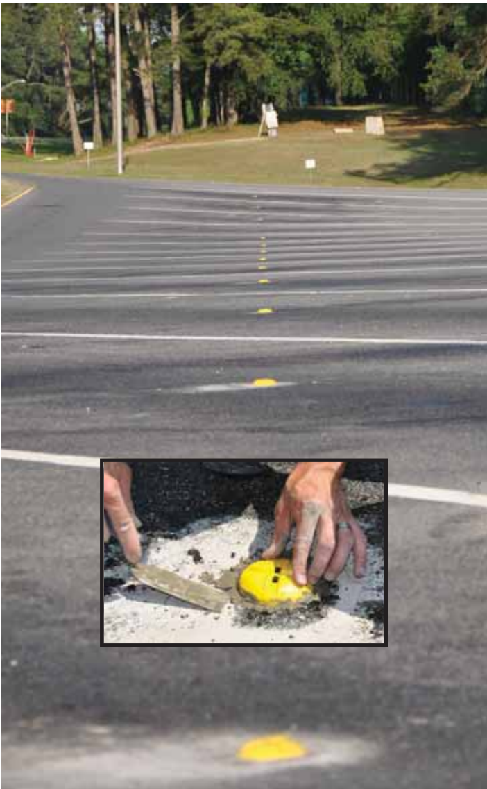
Above: Wireless occupancy detection sensors installed in truck parking spaces at the test rest area on I-10 in Leon County, Florida. Insert: A technician installs a detection sensor in the pavement.
