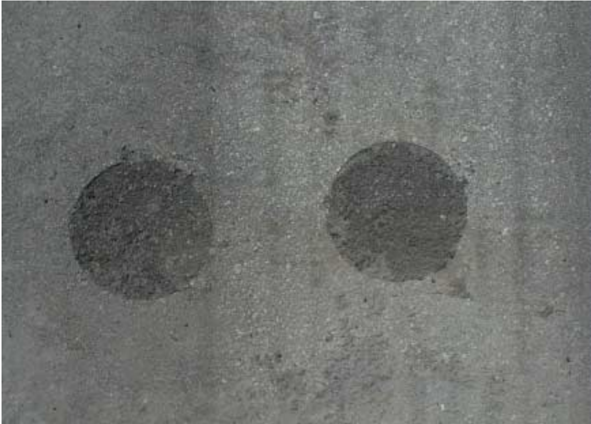
Figure 9.1 Picture Showing Locations of a Core Taken From the Middle of the Wheel Path and a Core Taken From the Outside Edge of the Wheel Path
