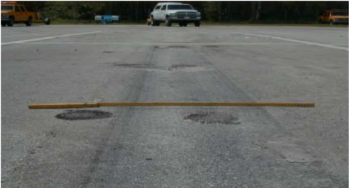
Figure 7.7 Photo of Section 3B (SBS-Modified Mixture over Unmodified Mixture Tested at 50° C)
