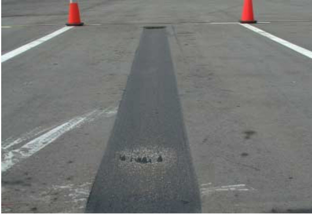
Figure 6.4 Section 5C (Unmodified Mixture) after HVS Testing
