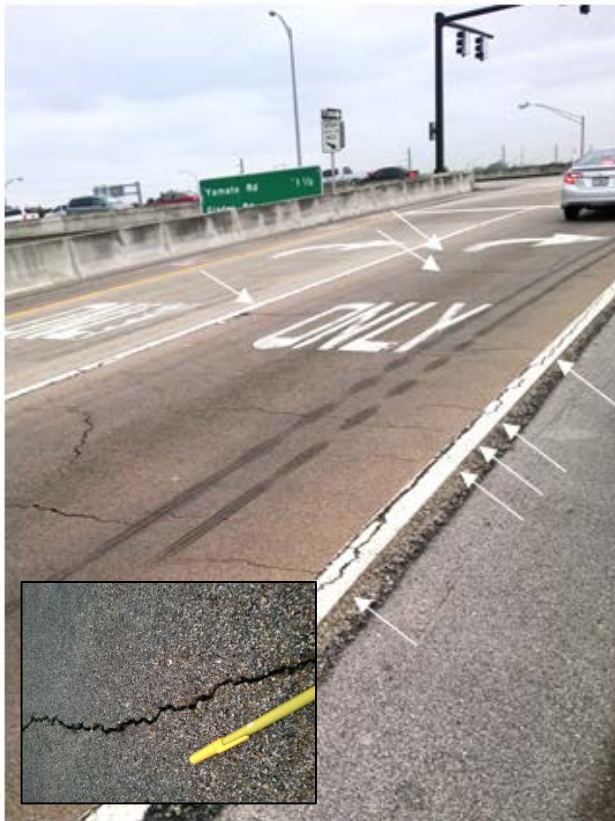
FIGURE 20 – Substrate top-down tearing at a signalized approach (transverse cracking).
