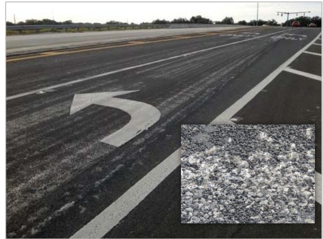
FIGURE 13 – Aggregate loss over uneven texture.
