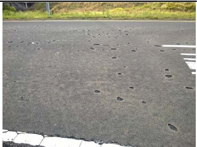
FIGURE 16 – Widespread localized failures due to poor binder mixing.
