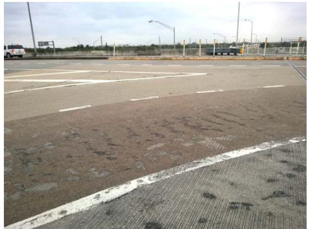
FIGURE 14 – Aggregate loss over concrete.
