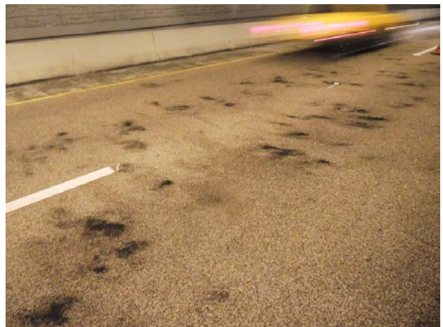
FIGURE 17 – Soft splotchy areas shortly after construction.
