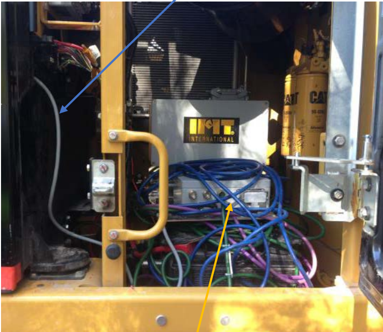
Junction box mounted near battery
