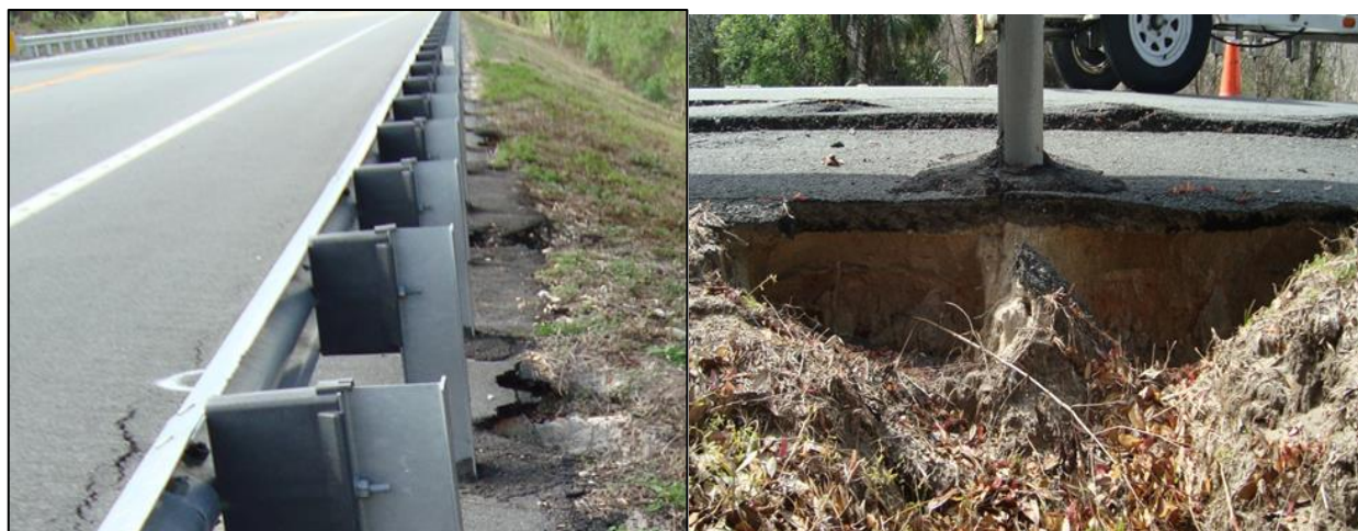
Figure 5 Unstable shoulder conditions
