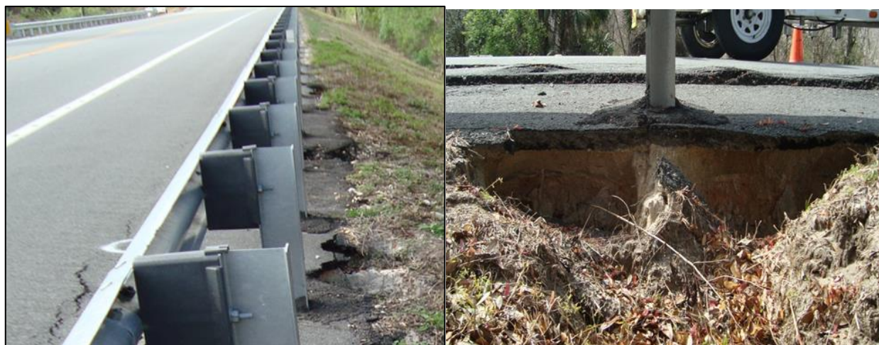
Figure 5 Unstable shoulder conditions
