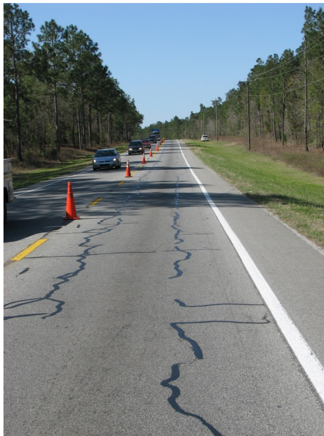
Figure 2 – Typical Representation of Cracking
