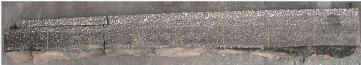
Figure 5 – Southbound Trench at Pavement Failure Area of CR-315 Project
