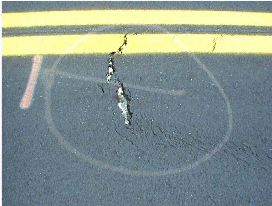
Figure 3 – Cracking and Delamination Damage for CR-315 Project
