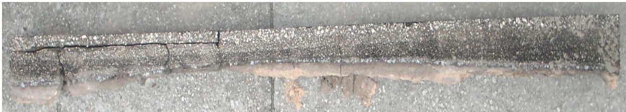
Figure 4 – Northbound Trench at Pavement Failure Area of CR-315 Project
