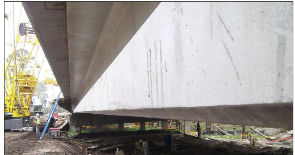
Pictured to the right, is a similar girder to the one above after deck casting – notice the relatively flat profile of the girder that has resulted because of the downward deflection caused by the deck load thus reducing the camber
