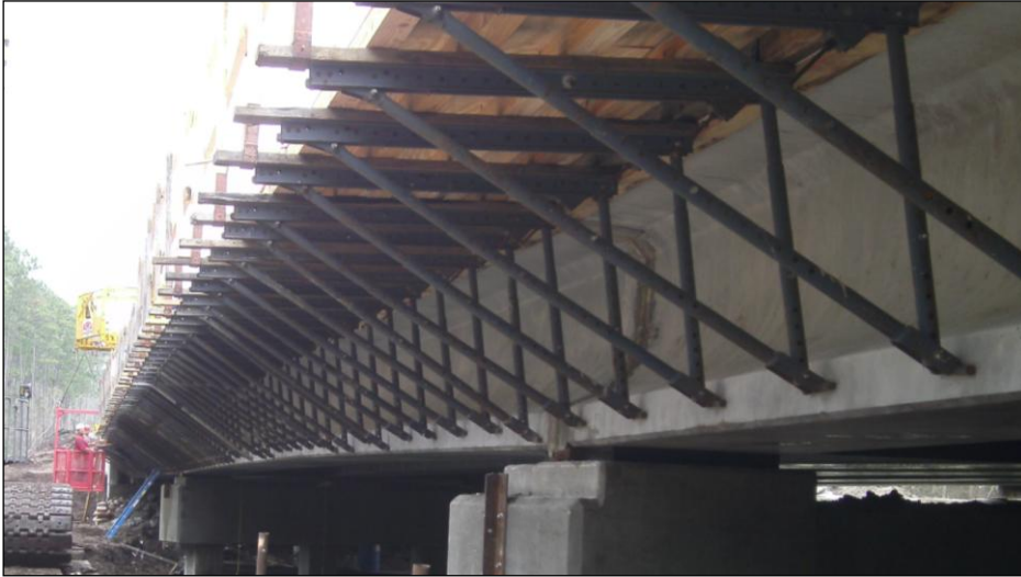
Pictured to the left, is a girder prior to deck casting – notice the slight upward curvature or camber of the girder
