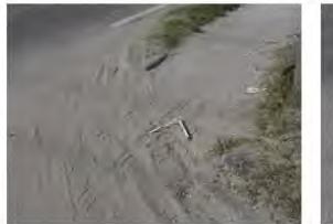
These pictures show example of sand buildup on sidewalk. Sweeping should be rated around the
