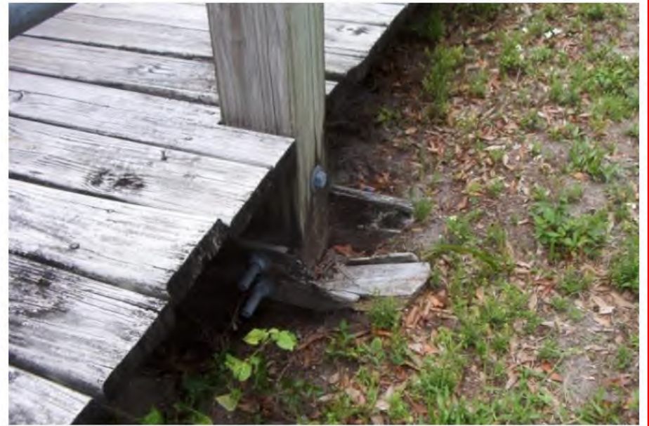
Deterioration of supports.
