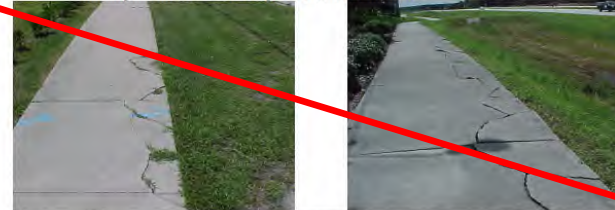
Sidewalk cracking. Measure each horizontal crack greater than \frac{1}{2} inch wide. For MRP purposes, each linear foot of horizontal crack greater than \frac{1}{2} inch equals 1 sq. ft. of crack area. Vertical misalignments greater than \frac{1}{4} inch equals 1 sq. ft. of crack area.
