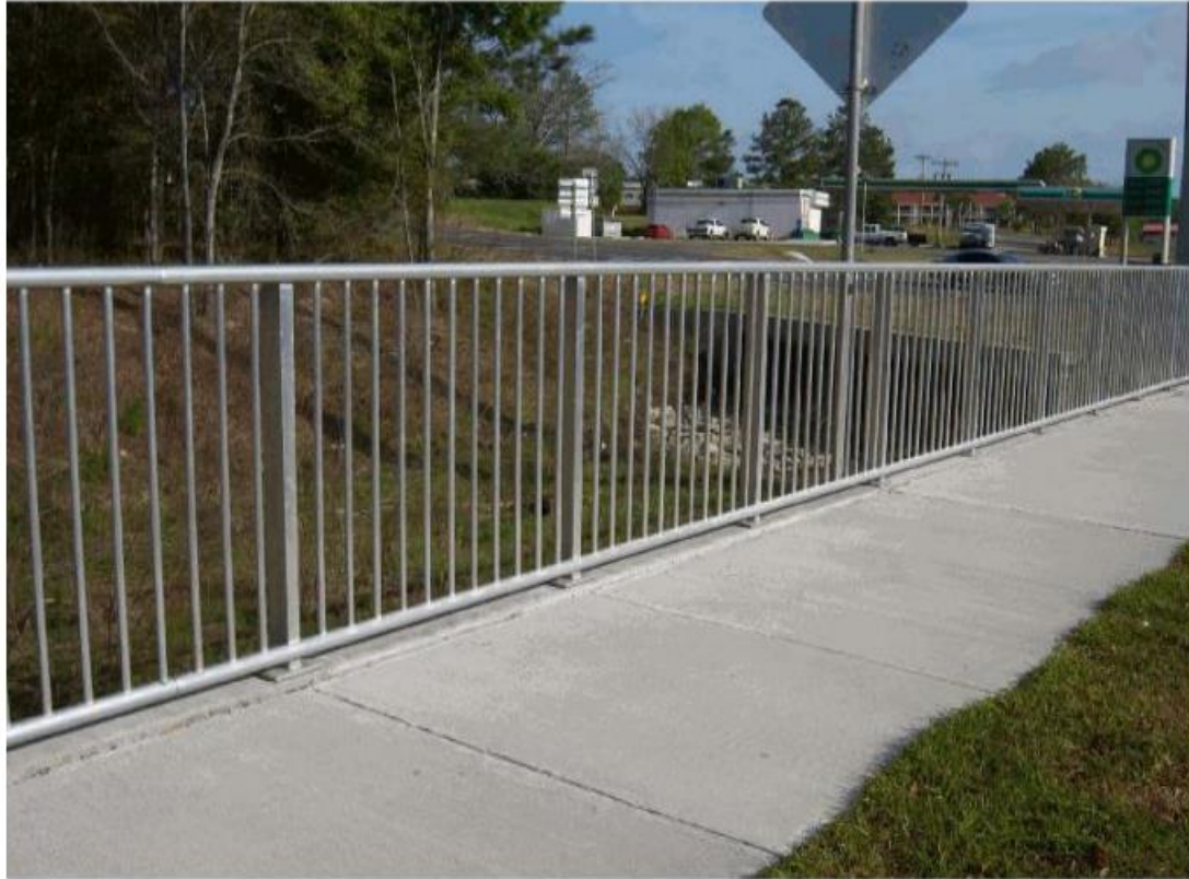
Picket railing protecting drop-off next to sidewalk.
