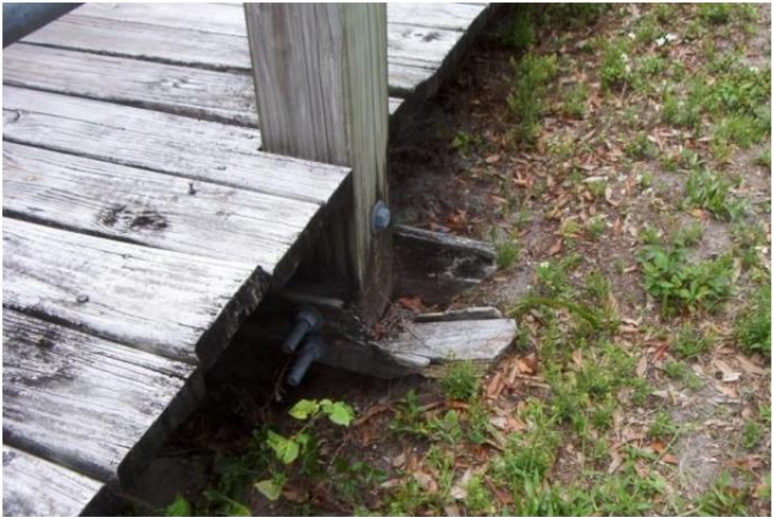
Deterioration of supports.
