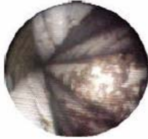
Figure 16, Borescope photo showing ungrouted stands
