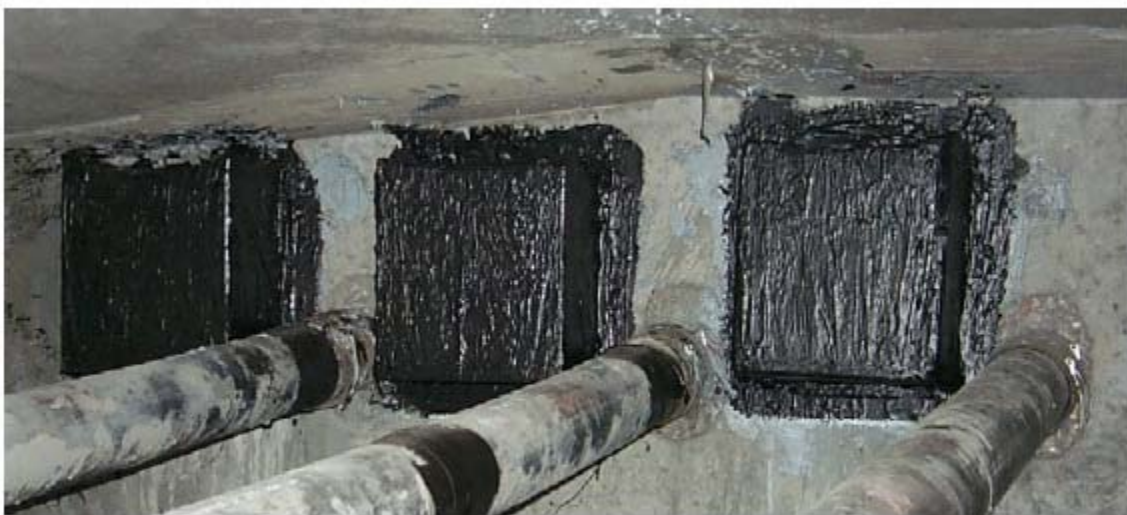
Figure 18. Anchorhead pourbacks for external tendons that exit the opposite side of the diaphragm
