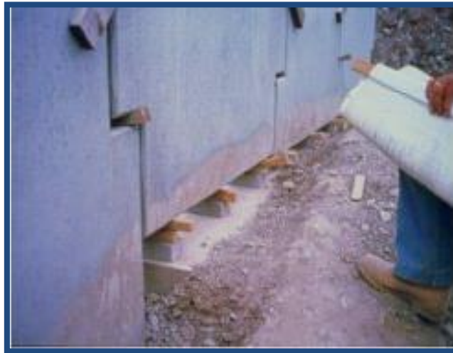
Figure 5-2: Improper Leveling Pad
