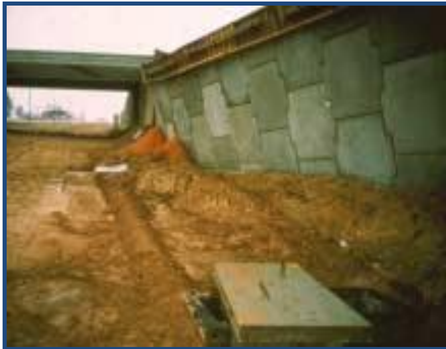
Figure 16-8: Wall Failure from Exterior Excavation
