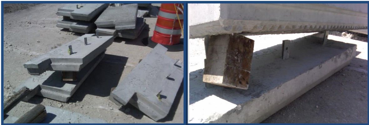
Figure 6-9: Improper Panel Storage
