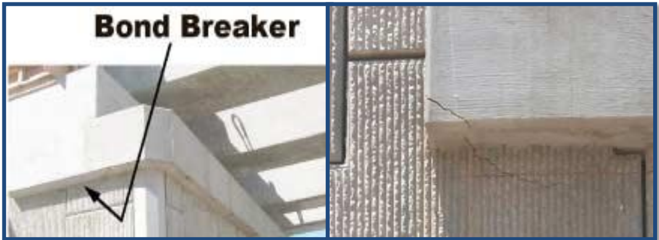
Figure 11-1: Bond Breaker (Left) and Cracked Panel/Cheek Wall (Right)
