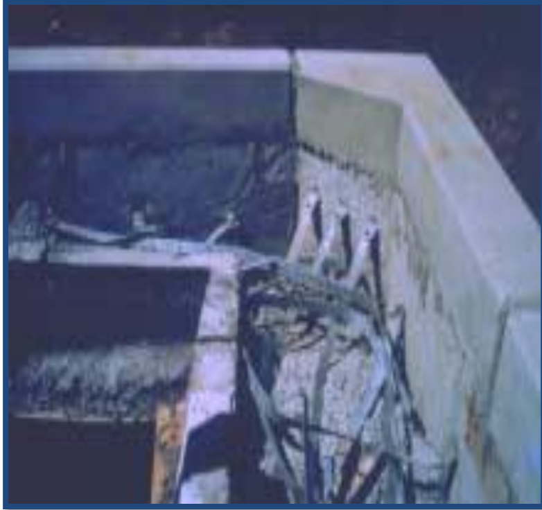
Figure 16-4: Improper Avoidance of Drainage Structure
