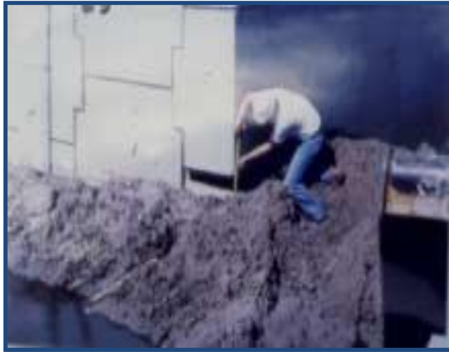
Figure 16-7: Joints Opening from Settlement
