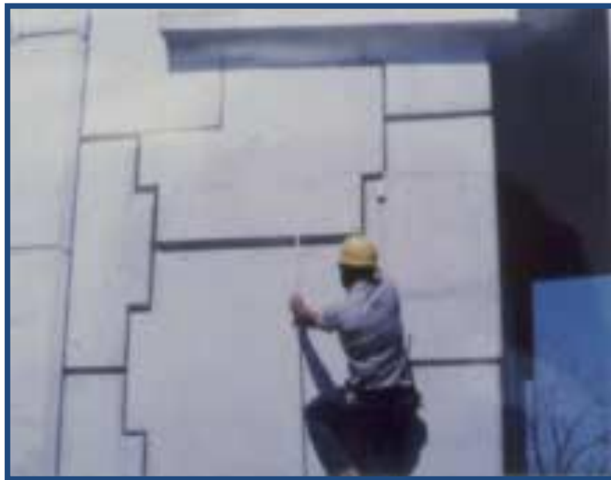
Figure 16-6: Settlement from Excavation
