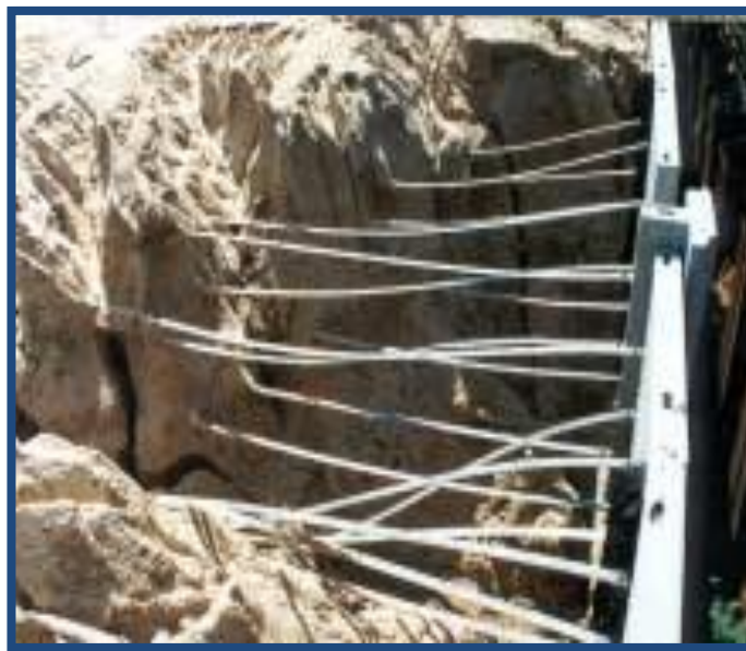
Figure 13-2: Wash Out from Around Reinforcement
