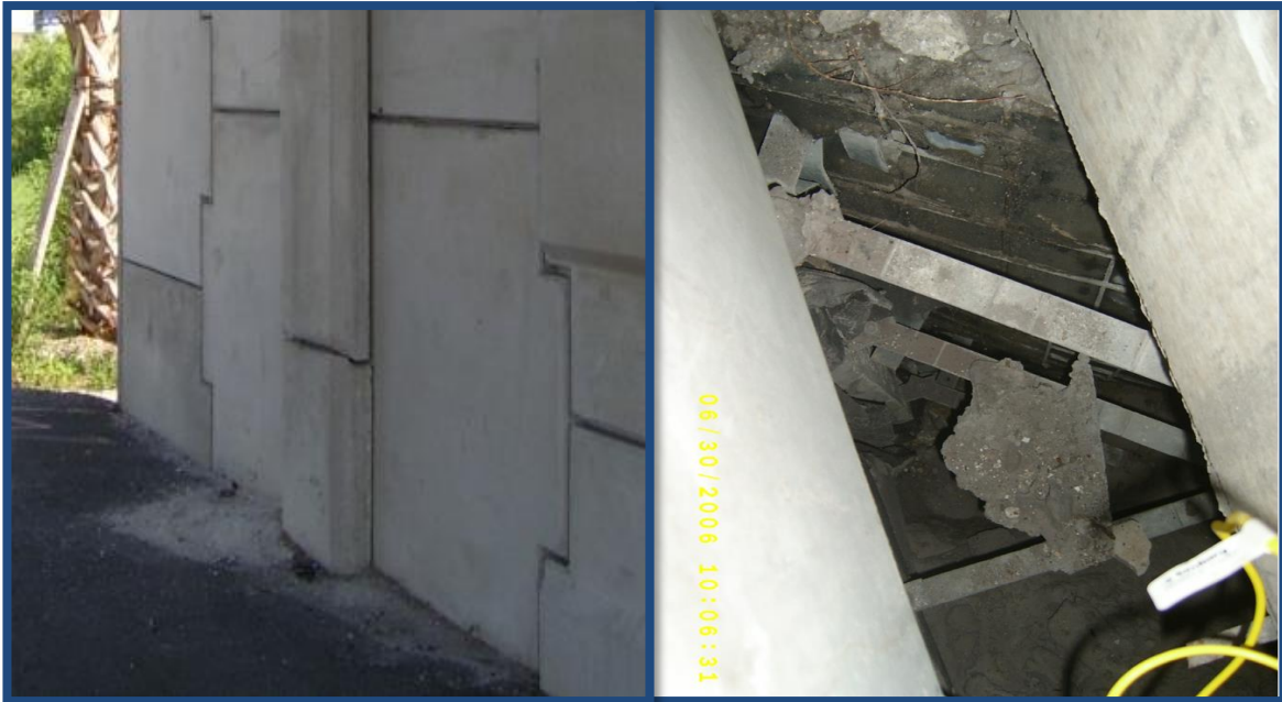
Figure 8-2: Loss of Backfill Through Improperly Constructed Joint and Filter Fabric
