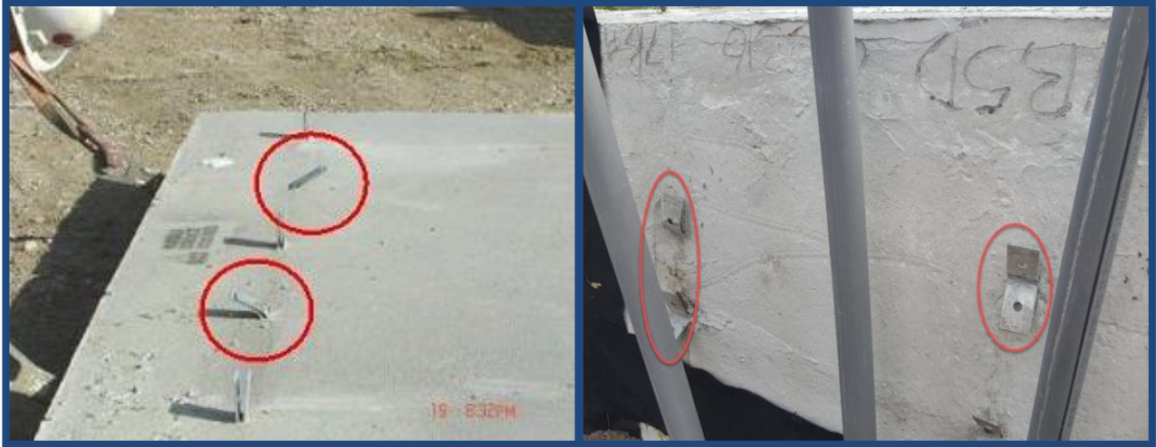
Figure 6-10: Damaged Panel Tabs
