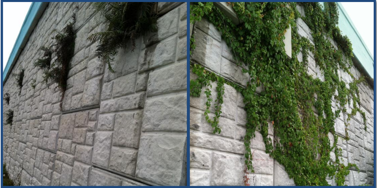
Figure 9-1: Vegetation Growth in Joint Openings
