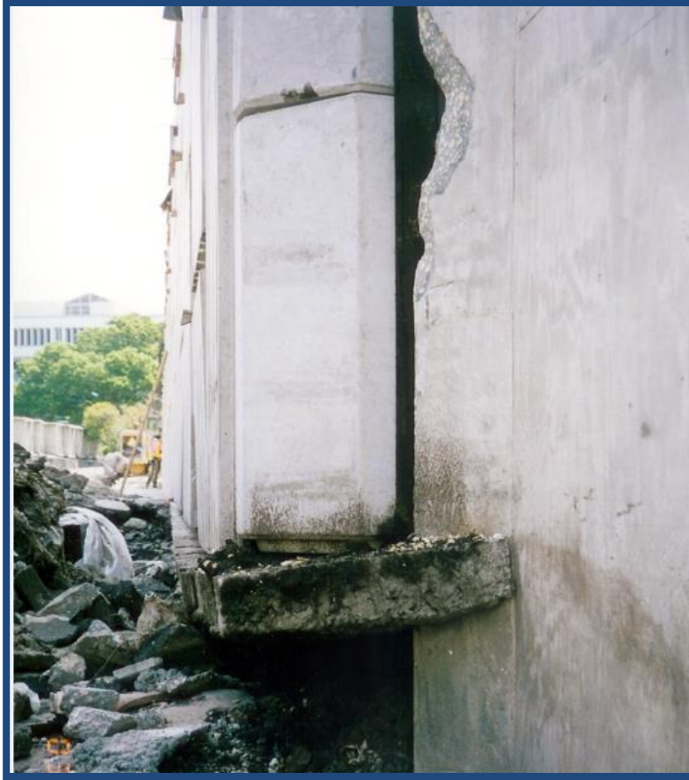
Figure 13-3: Undermining Leveling Pad
