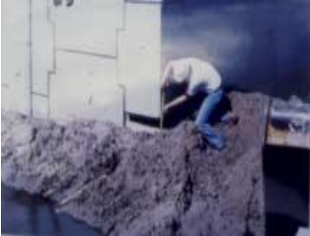
Figure 37, Settlement from Excavation
