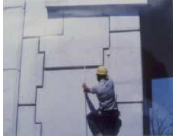
Figure 38, Joints Opening from Settlement
