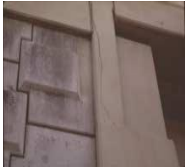
Figure 31, Tension Break in Cheek Wall
