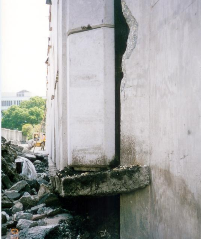
Figure 34, Undermining of leveling pad
