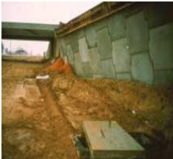
Figure 39, Wall Failure from Exterior Excavation
