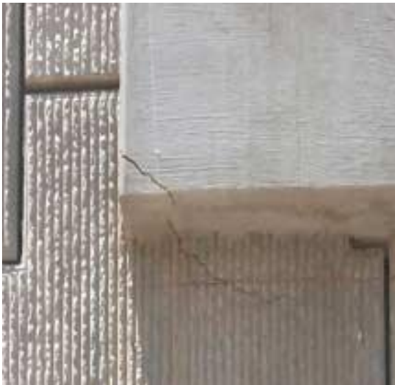
Figure 30, Cracked Panel and Cheek Wall
