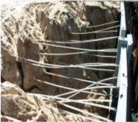
Figure 33, Wash Out From Around Reinforcement
