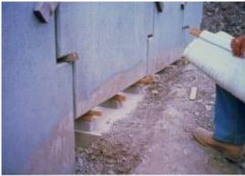
Figure 4, Improper Leveling Pad
