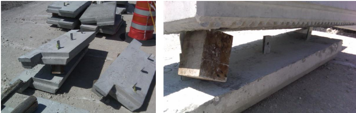
Figure 14, Improper Panel Storage
