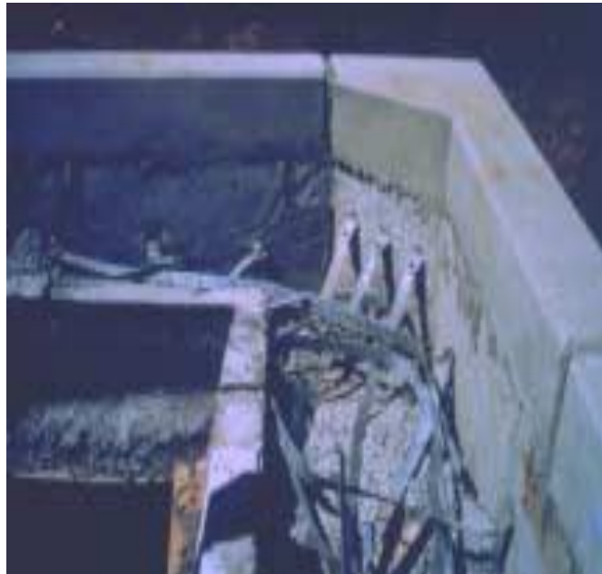
Figure 36, Not Proper Avoidance of Drainage Structure
