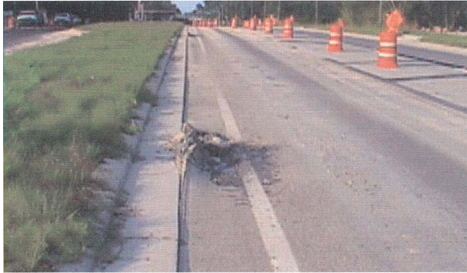
Exhibit 1 – Failure of old mix design asphalt.
