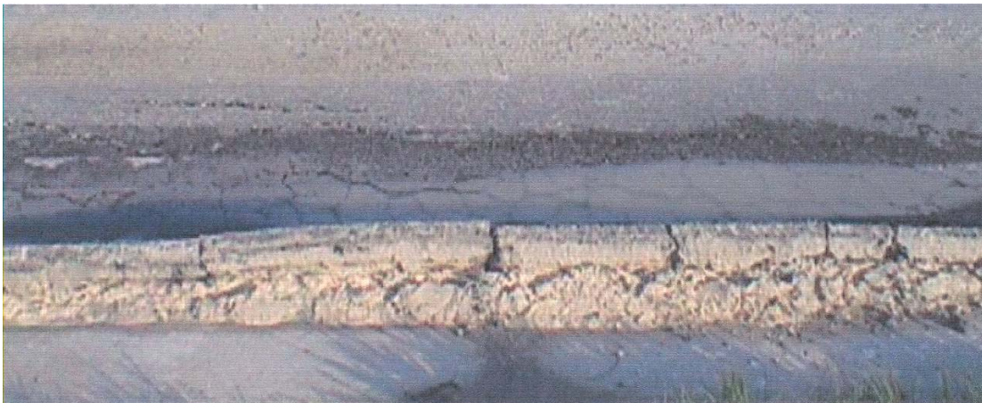
Exhibit 5 – Failed old design mix roadway
