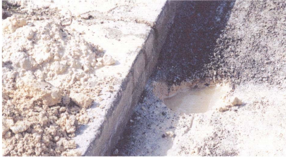
Exhibit 3 – Water seeping under curb from median
