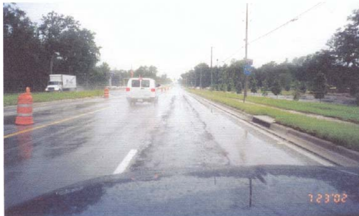
Exhibit 4 – Patched old design mix due to previous failure.
