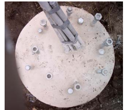
Unsatisfactory drilled shaft
