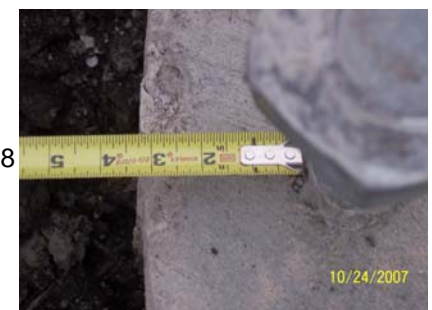
Insufficient concrete cover
