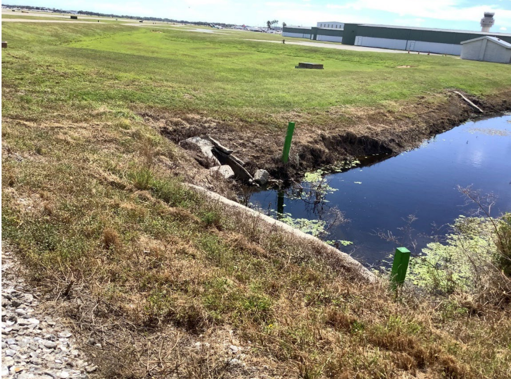
Figure 701-7 Inlet Structure Requiring Maintenance
