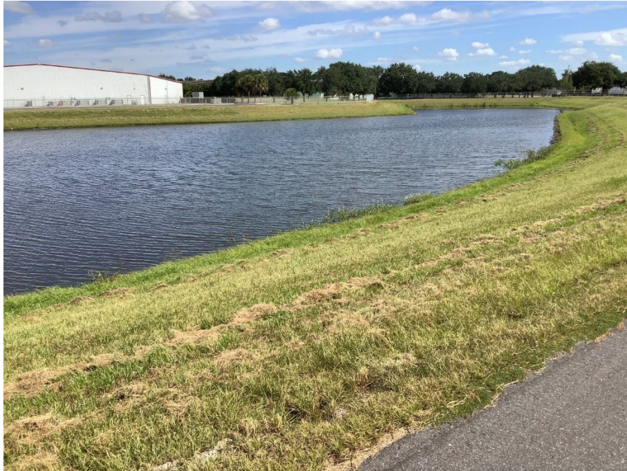
Figure 701-1 Well Maintained and Functioning Wet FAA Pond
