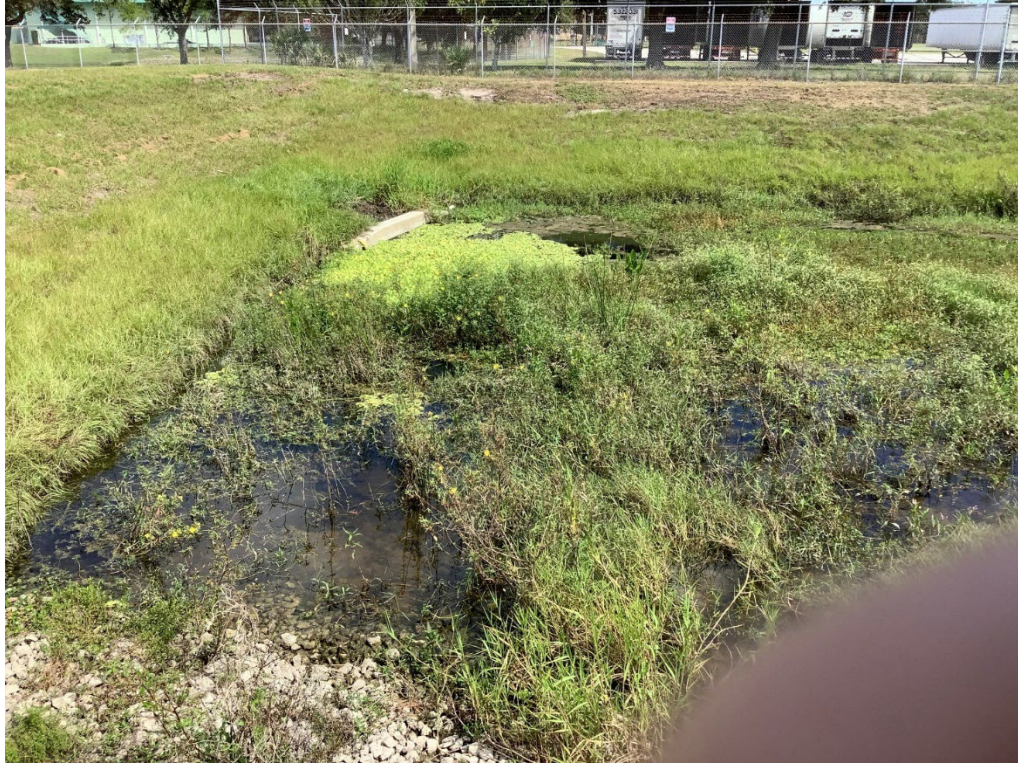
Figure 701-5 Clogged Inlet Pipes
