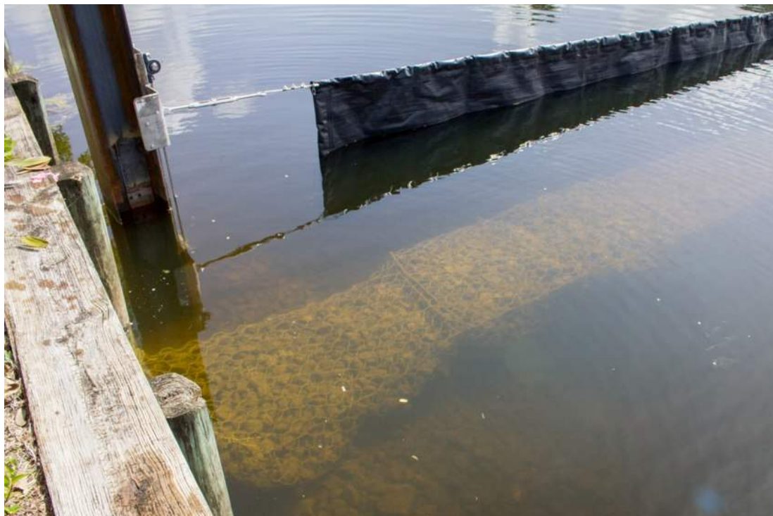
Figure 7 – Moveable Fabric Baffle and Fixed Gabion Baffle. Fabric is Up-Gradient.
