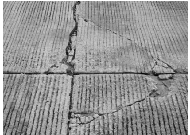
▶ Corner cracks with spalling. Full depth patch required.
