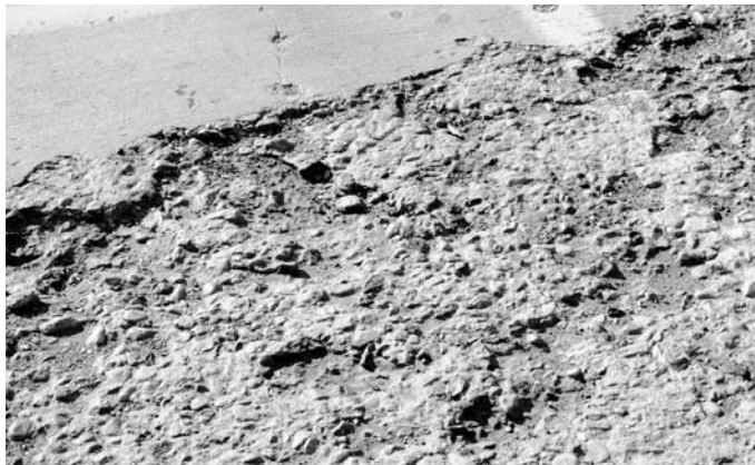
► Moderate surface scaling. Loss of mortar and fines starting to expose larger aggregate.
