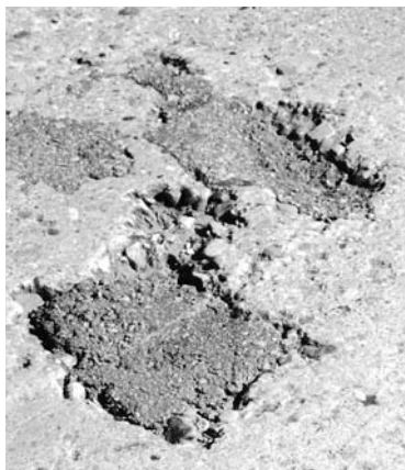
◀ Small surface spall that has been patched.
