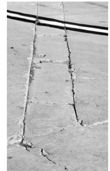
▲ Concrete patch in poor condition.
