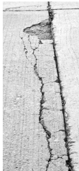
▲ Full depth joint repair required.
