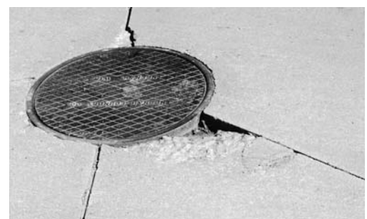
▼ Two spalls at manhole in a new pavement. Partial depth patching would be beneficial.
