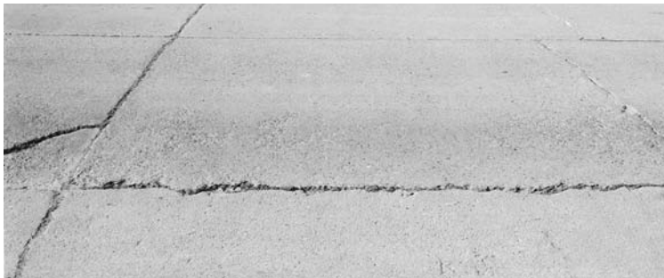
▼ Open cracks with edge spalling. Corner crack and broken corner piece.
