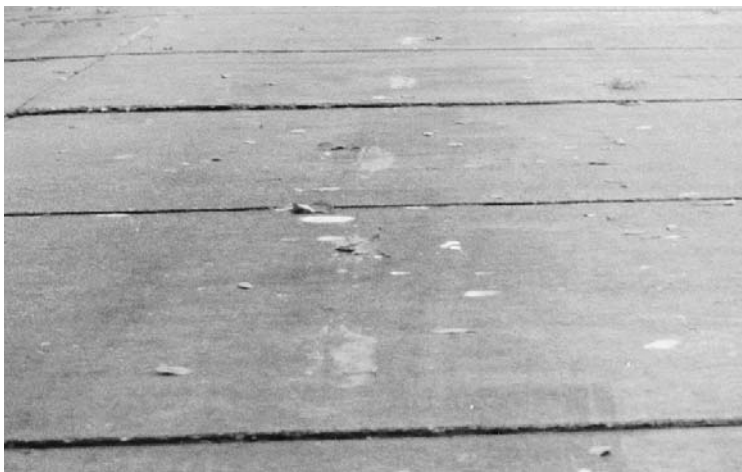
▲ Faulting of joints aggravated by heavy traffic in one direction.
