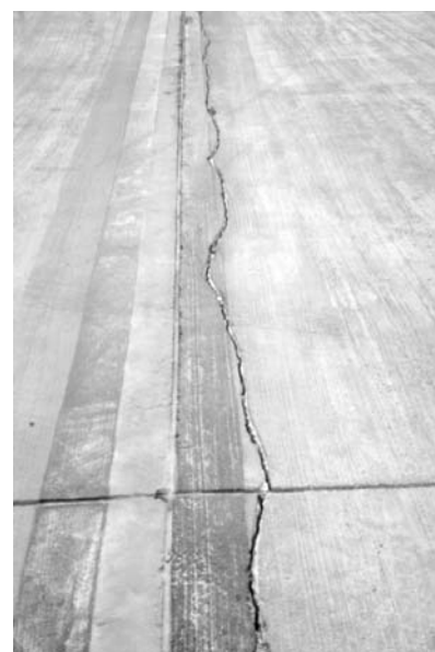
◀ Crack parallel to joint. Open 1/4". No spalling.
