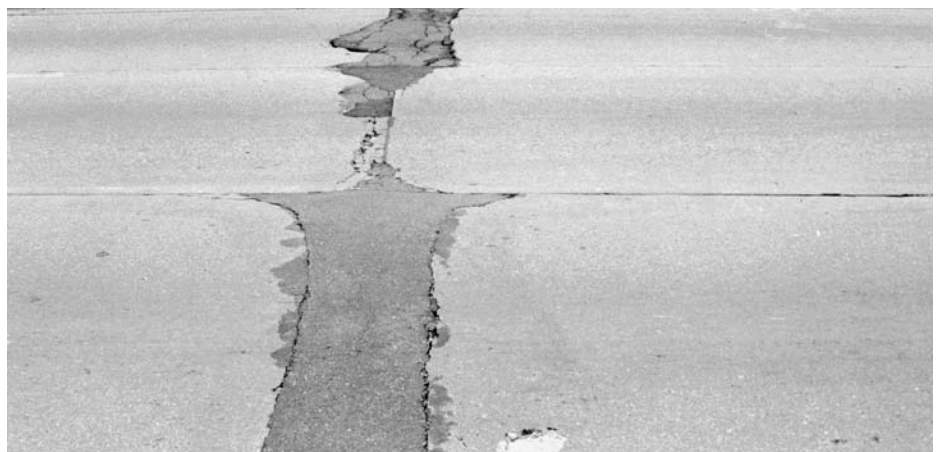
▶ Asphalt patches. Poor (top) and fair (bottom) condition.
