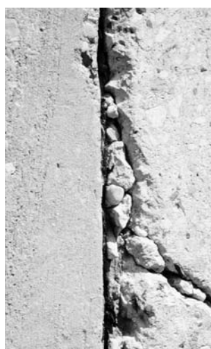
▲ Severe spalling along joint and crack. Creates debris.
