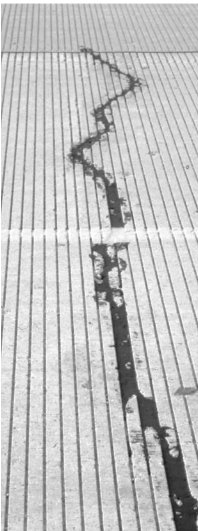
▲ Crack breaks slab into two pieces. Well sealed.
