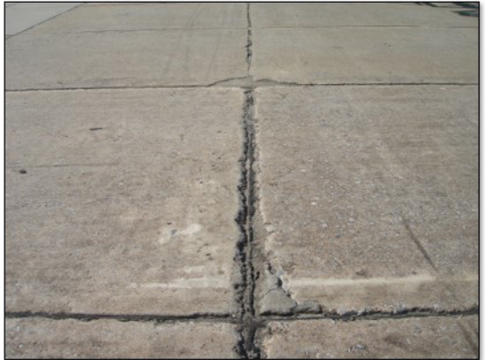
Joint Seal Damage
