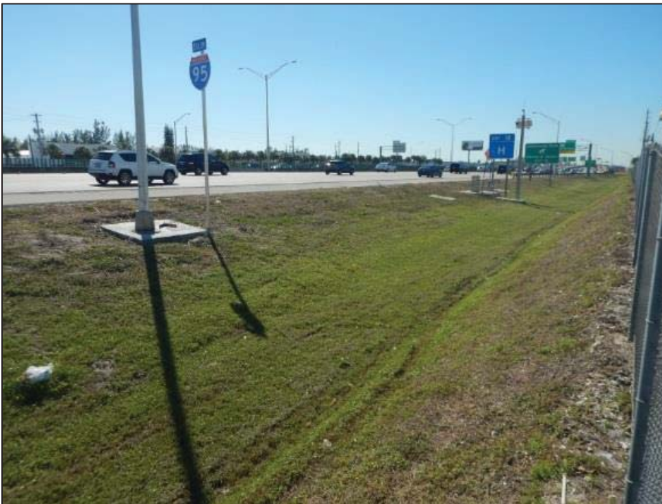
Photo 4: Swale-3 on the west side of I-95 between Pembroke Road and Hallandale Beach Boulevard.
